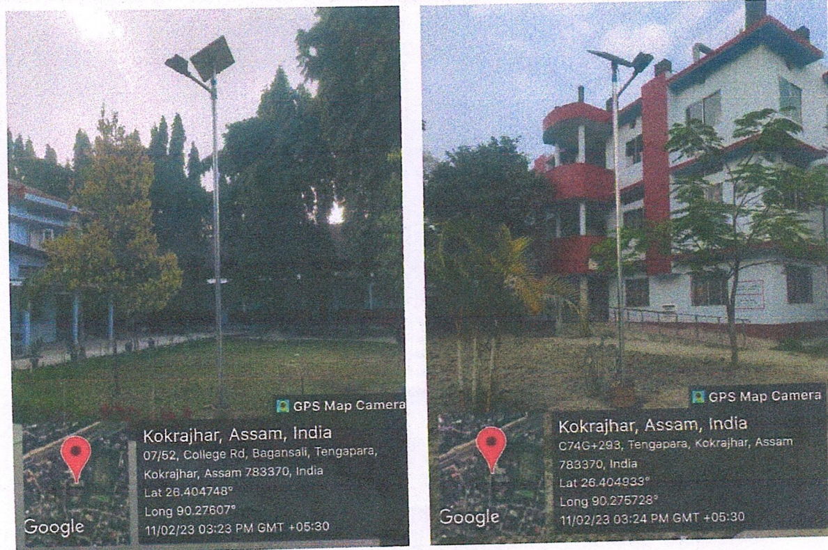
Figure 9: Solar Street light installed in the campus
